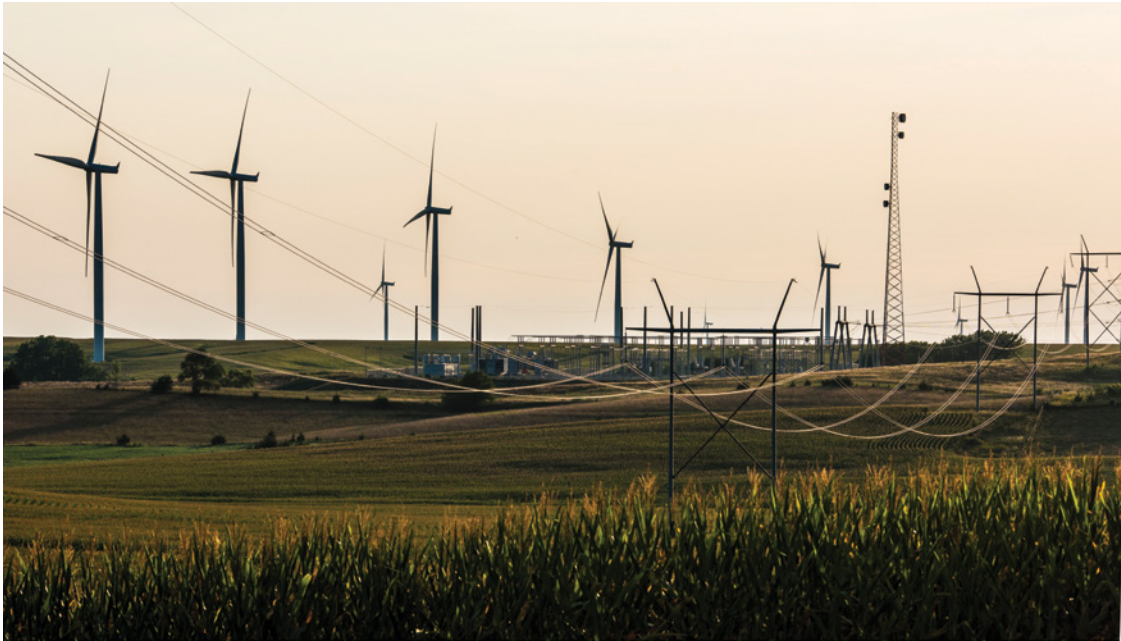
FIGURE 10.5 A cluster of wind turbines
